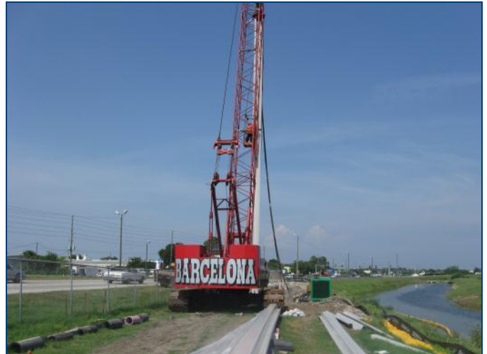
Vinyl sheet piling was installed using a vibratory hammer, not unlike installing steel sheet piling.
