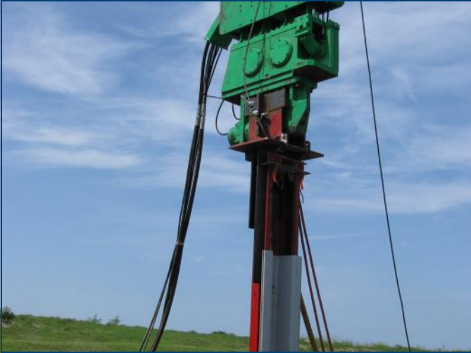
A steel mandrel was used to aid in penetration through resistant materials.
